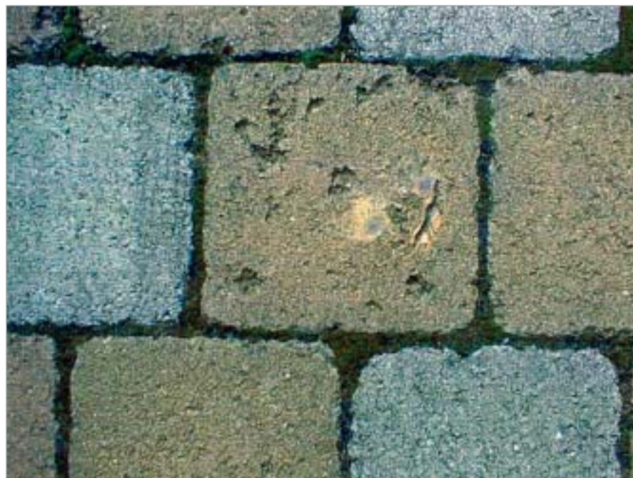
Figure 20: Paving stone with washed out pigment, laid 1997
