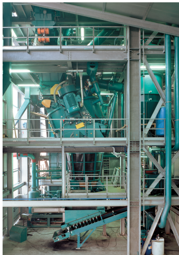
Fig. 4.1: Eirich sand preparation system with EvacTherm® RV32VAC mixer-cooler
