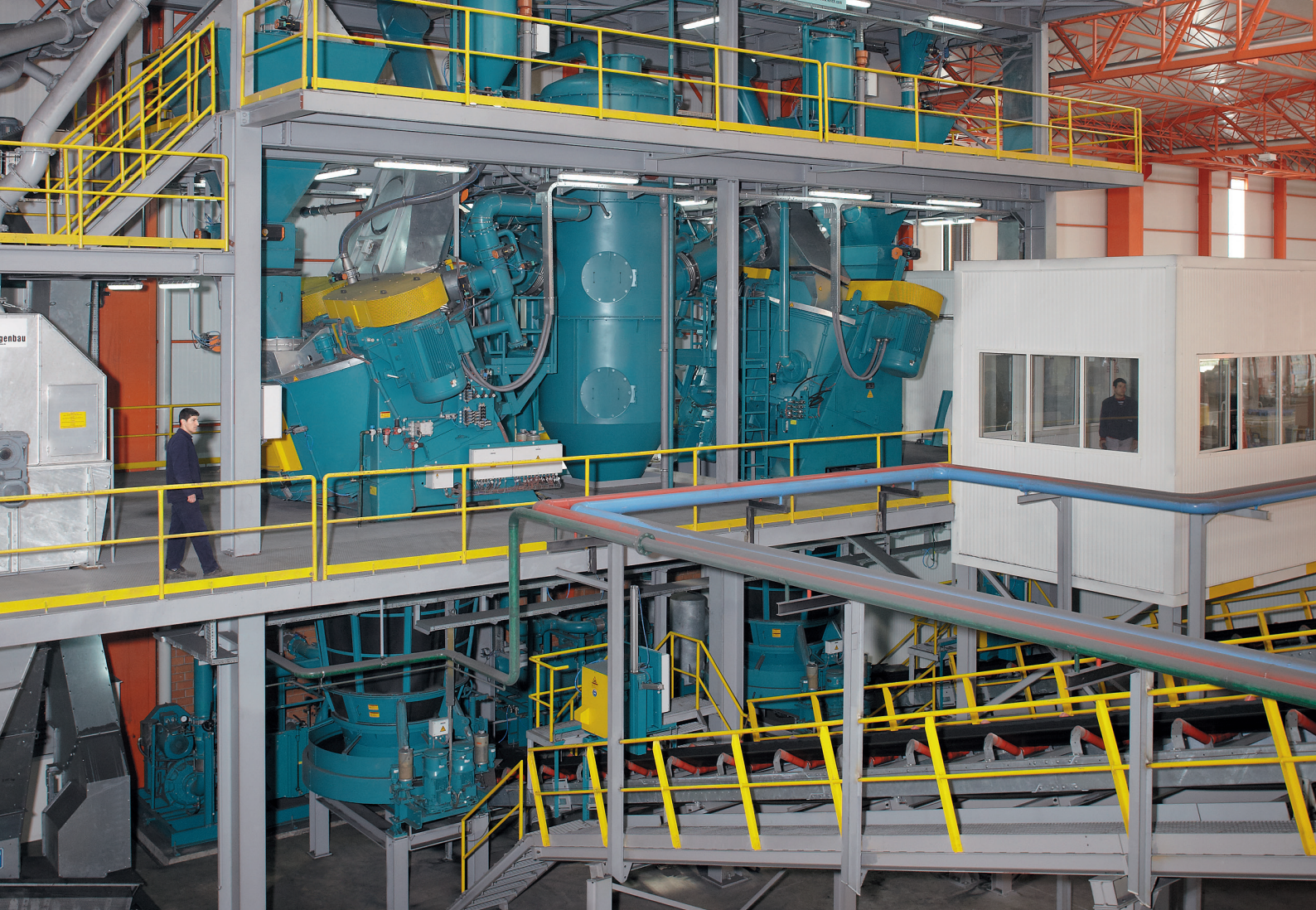
Fig. 6.1: Two EvacTherm® RV32VAC mixer-coolers (7 m 3 = 247 ft 3 per batch) for roughly 260 t/h (286.6 short tons/h) production demand.
