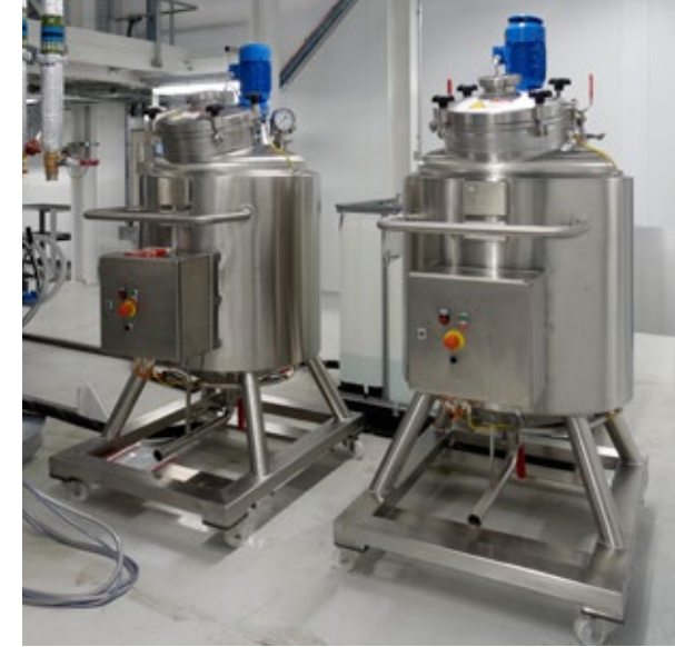
“Batch-pure” tanks in a pilot system
