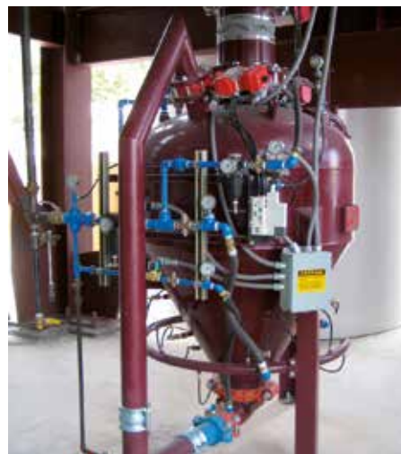
Pneumatic conveying system
